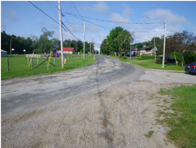
Image 1: View of disturbances associated with the paved roadway of Warminster Sideroad, gravel shoulders, buried utilities (hydro, watermain and gas main) and paved driveways.
