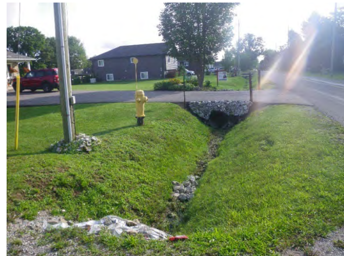
Image 8: View of disturbances associated with buried utilities (hydro and watermain), roadside ditching and paved driveway.
