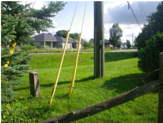
.Image 15: View of disturbances associated with buried utilities (telecommunication wires, hydro and gas main).
