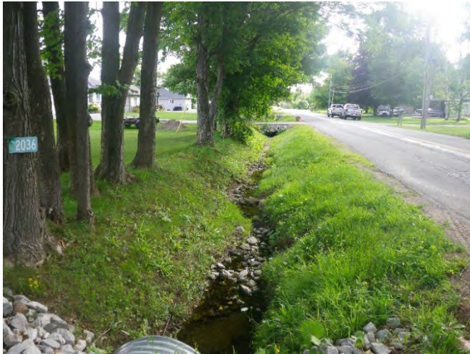
Image 5: View of disturbances associated with deep roadside ditching.
