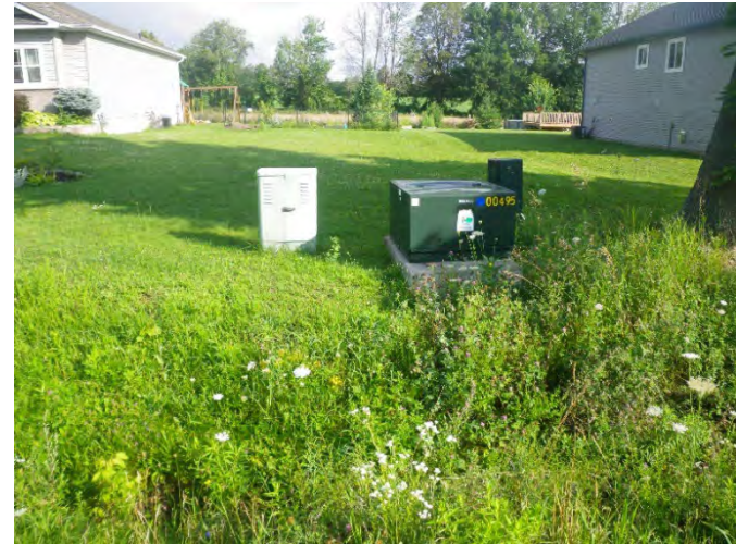
.Image 14: View of disturbances associated with buried utilities (telecommunication wires).
