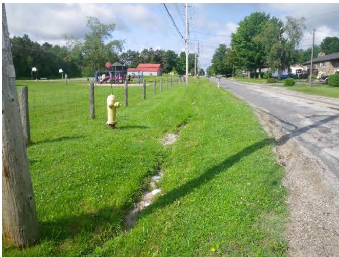
Image 11: View of disturbances associated with buried utilities (hydro, watermain and gas main), roadside ditching and paved roadway.
